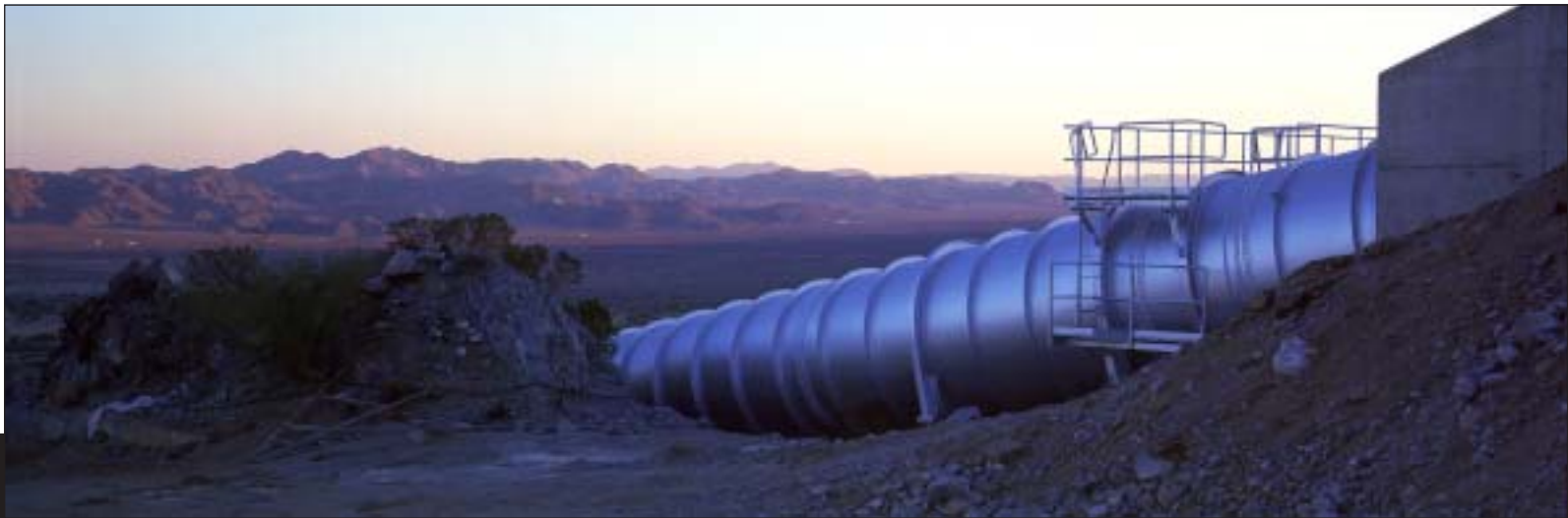
L.A.-bound water from the Colorado River is pumped uphill through one of three metal pipes in the high desert
